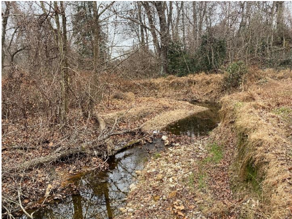
Incised and widening channel beginning to encroach on the sewer.
