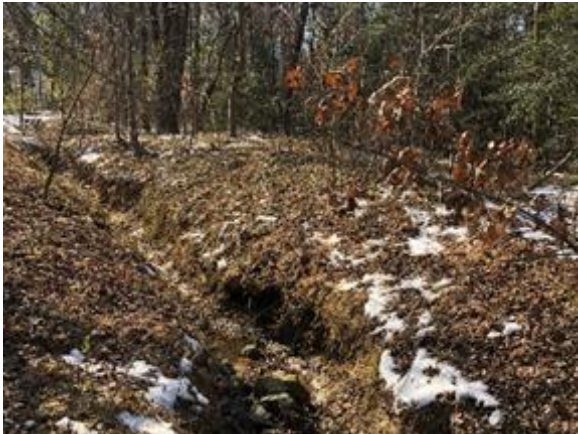
Degraded outfall channel.
