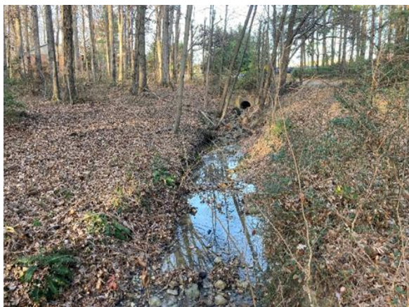
Incised and widening outfall channel.
