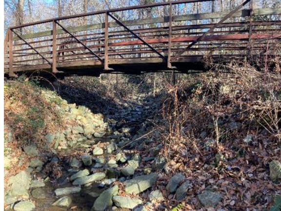
Large pedestrian foot bridge spanning stream where elevation and plan form are a constraint.
