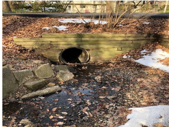
Undersized culvert downstream beneath private driveway.
