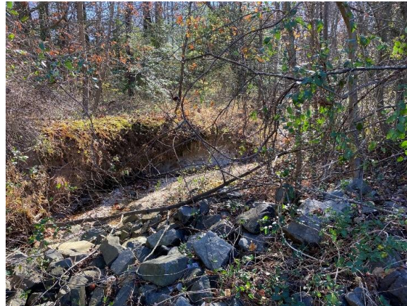
Degraded outfall channel.
