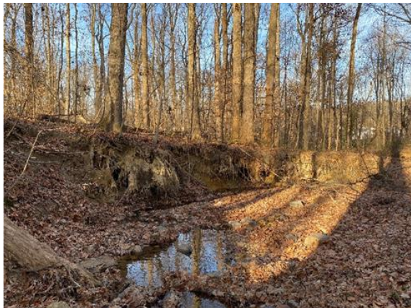
Incised and widening channel.
