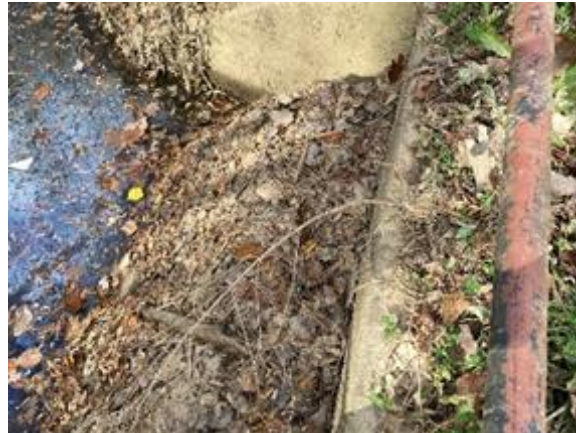
Clogged low-flow orifice.
