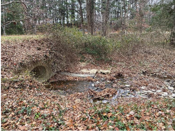
Exposed sewer encasement.
