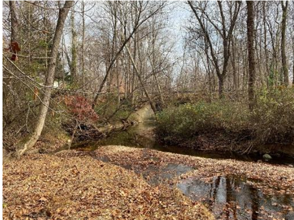
Widening stream channel with poor alignment into downstream culvert; large supply of sediment and streambed material in front of two culvert openings.
