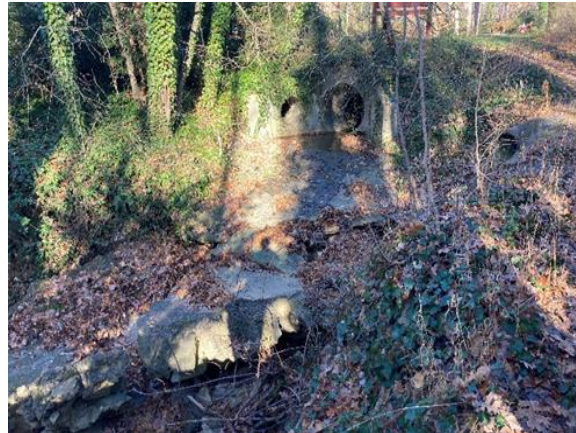
Three outfalls at upstream end of reach with failing apron structure.
