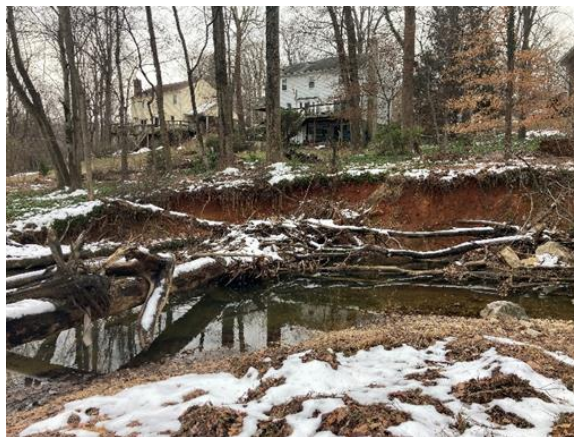
Stream channel impeding on private property.
