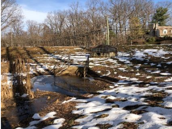
Backwatered trickle ditch and circular trash rack.
