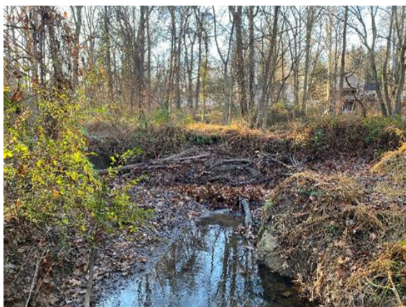
Debris blockage and exposed sewer manhole.
