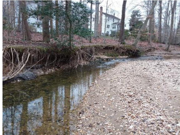
Widened stream channel with active bank erosion and an alignment nearing private properties.
