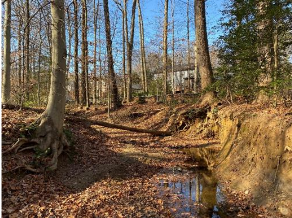
Widening channel with actively eroding banks near private properties.
