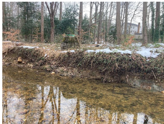
Channel alignment impeding on existing sewer infrastructure.
