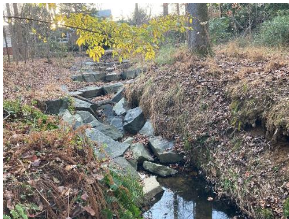
Previously stabilized outfall channel with grade control failure.
