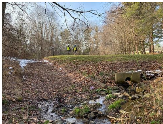
BMP-02 outfall and emergency spillway discharges into stream segment 0065-009.
