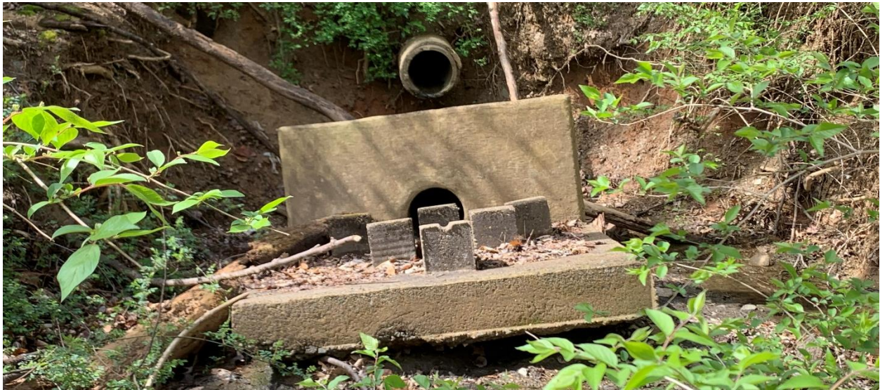
Collapsed outfall behind racquet club
